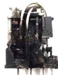
Burn damage due to insulation failure
