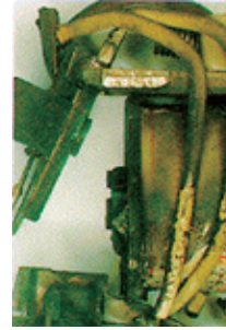
Burn damage due to overcurrent/overvoltage
