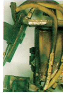
Burn damage due to overcurrent/overvoltage
