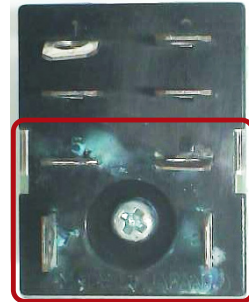
Deterioration of insulation in relay external terminal
