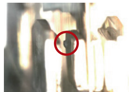
Contact transfer due to surge voltage
